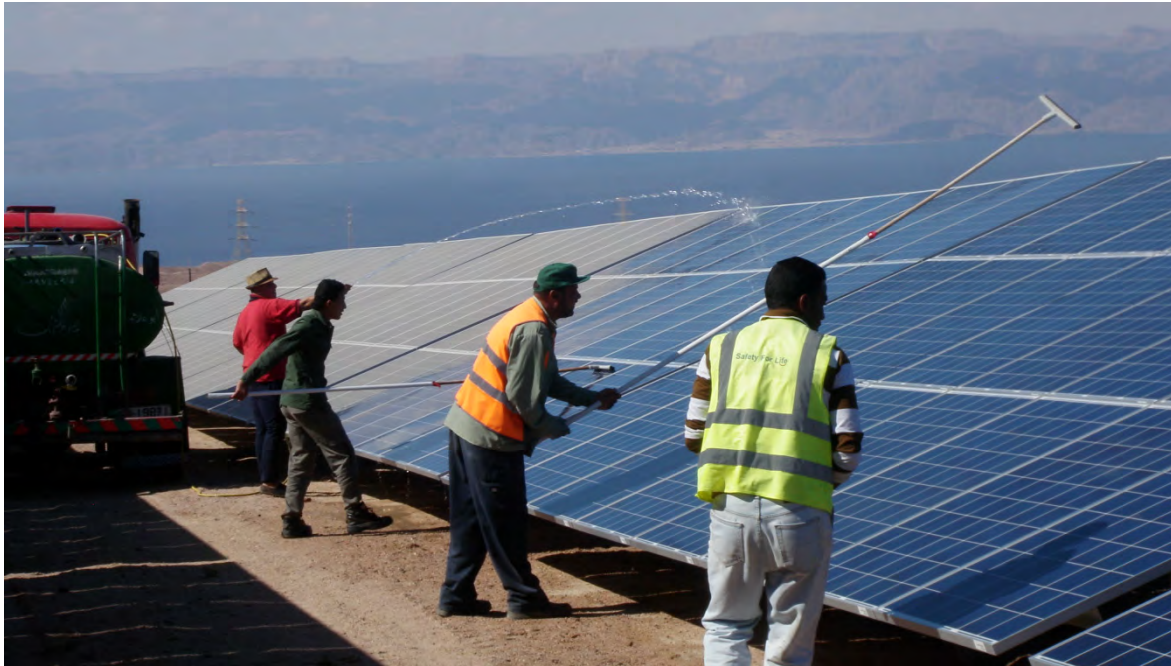
Fig. 35: Manual cleaning of a PV array. Photo: TÜV Rheinland Group
