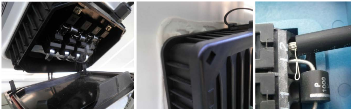
Fig. 6.1.3: Junction box failures: Left photo shows an open junction box in the field, the middle one a poorly bonded JB on the backsheet, and the right one a JB with poor wiring.
